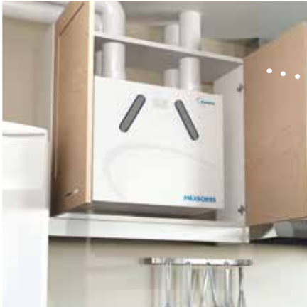
▲ (Model: MRXBOX95AB-WH2). Heat recovery unit mounted in a kitchen cupboard.
